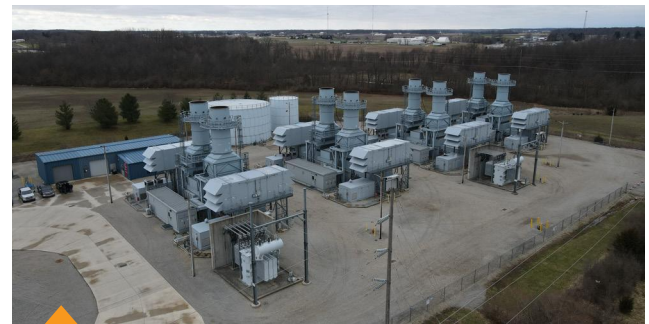
Greenville Generating Station Greenville, Ohio | 200 MW capacity
